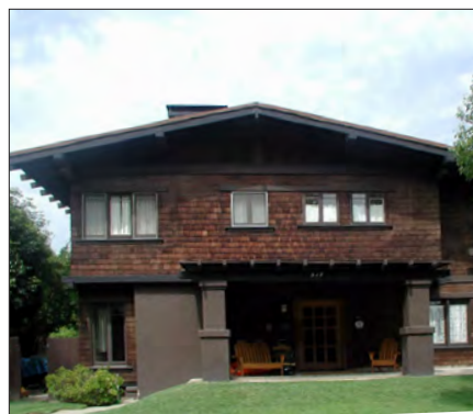
Unpainted siding above painted plaster
